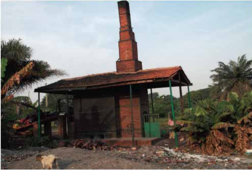
Figure 36: Medical waste incinerator in Ghana. Source: Adama, Esena et al. (2016)
