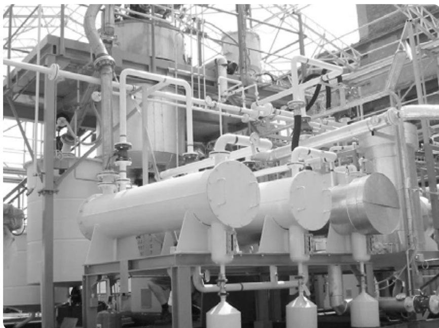
Figure 31: BCD destroyed POPs as second processing step in Spolana Neratovice, Czech Republic. Source: Kubal, Fairweather et al. (2004).
